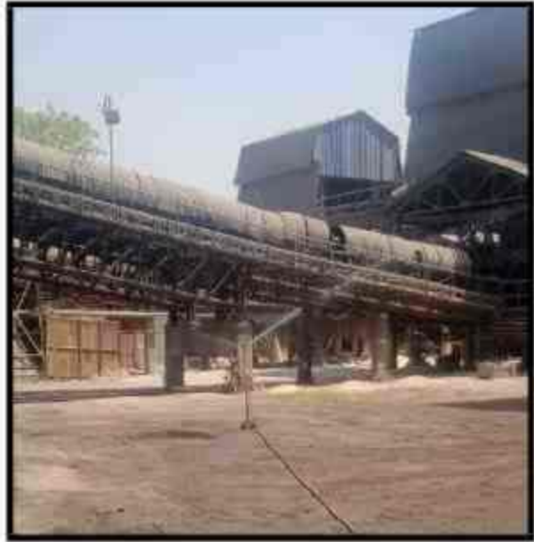
Belt conveyers are fully covered
