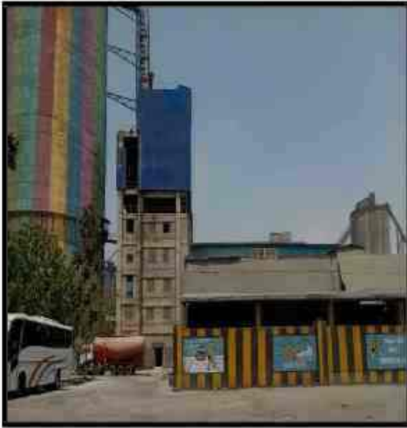
Covered packing unit
