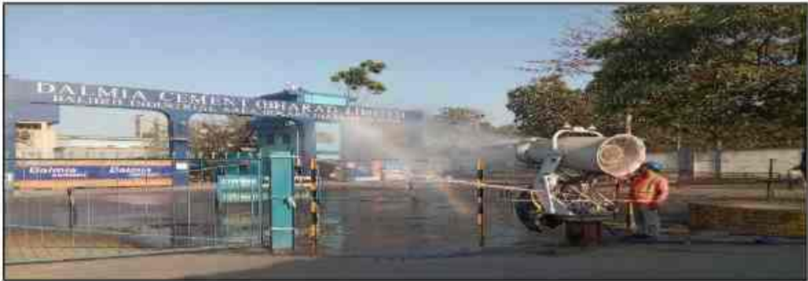
Water fog system installed in plant main gate
