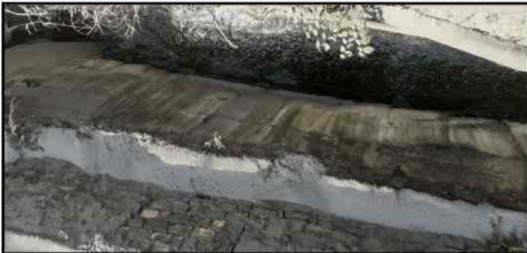
Rain water collection settling pit
